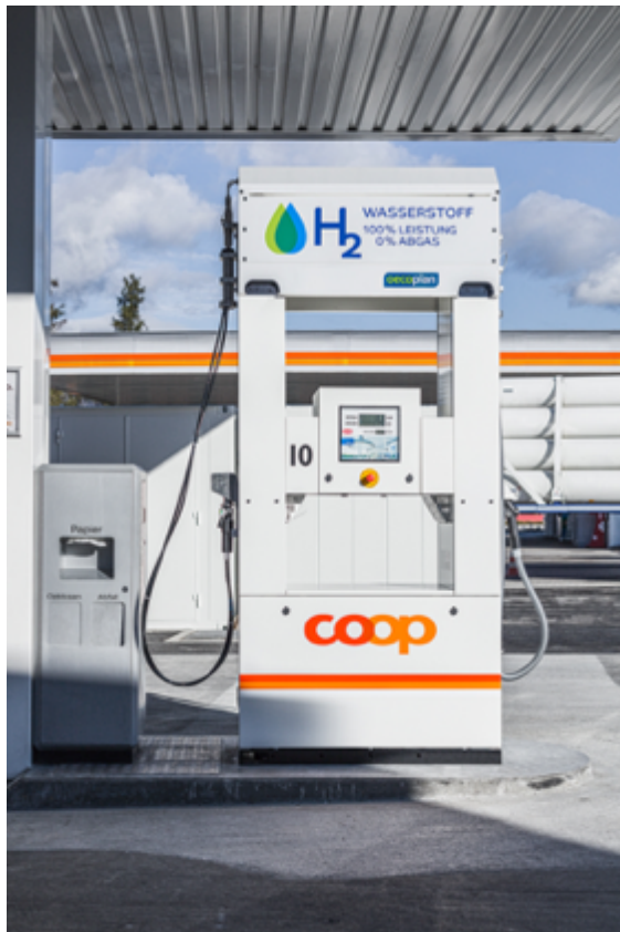
Coop HRS with H 2 Energy Trailer in the background
