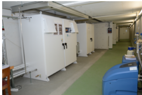
H 2 Energy electrolyzer and trailer refilling station
