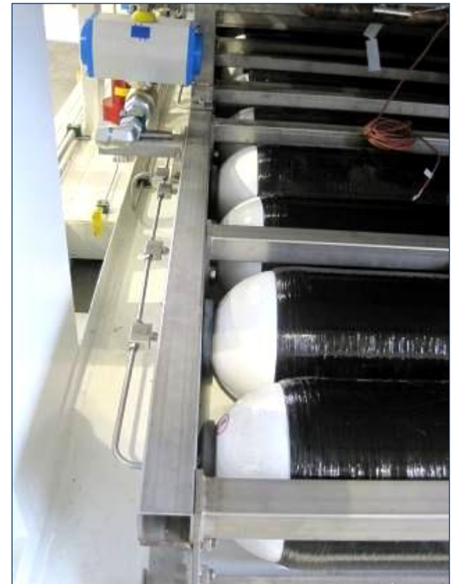
Fig. 2: Installed bottles – EU standard station
